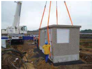
Inverter and transformer
