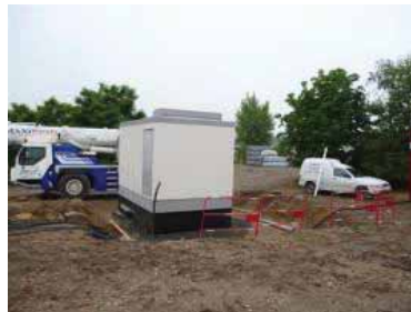
Medium voltage transmission station
