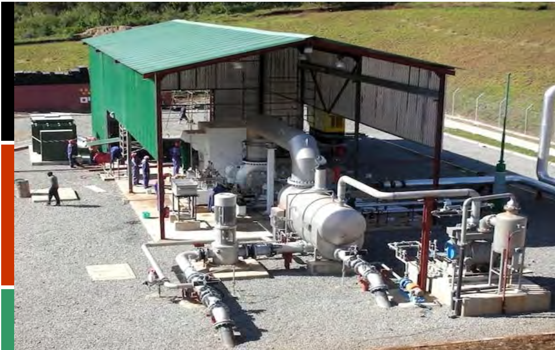
Plate 4: The 2.4 MW wellhead generator at the Eburru geothermal field
