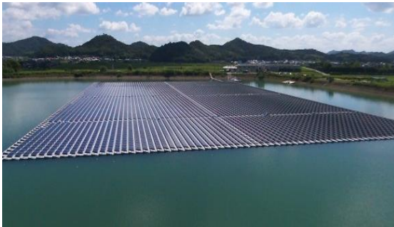
New solar PV plant (ground mounted or floating)
