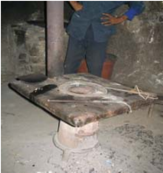
Figure 3.2a: Coal Iron Stove (left) and Chimney (right), Guizhou
