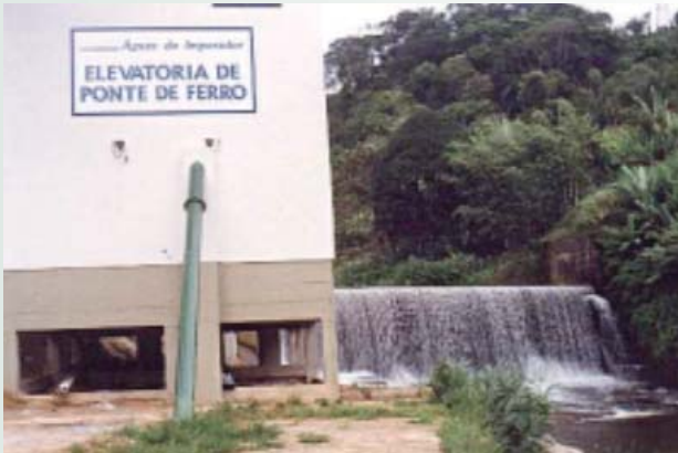
Ponte de Ferro water intake
