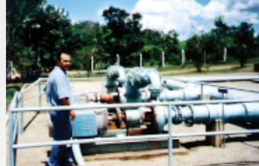
Palmas booster pumping station
