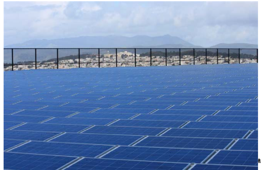
Sunset Reservoir – 5MW (2010)
