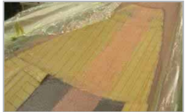
Spar Cap Grounding
