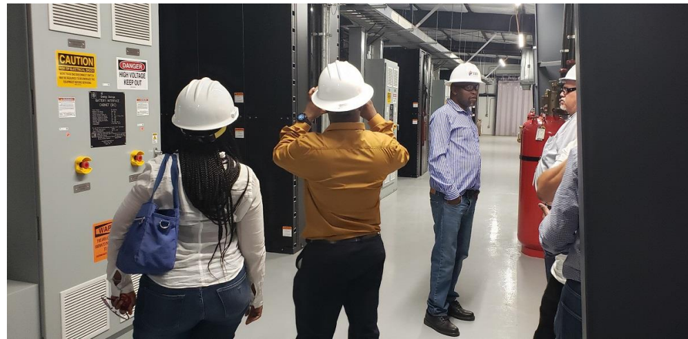
DPE / Eskom / DEA visit to IID Utility's 30MW Li-ion battery (San Diego, June 2019)
