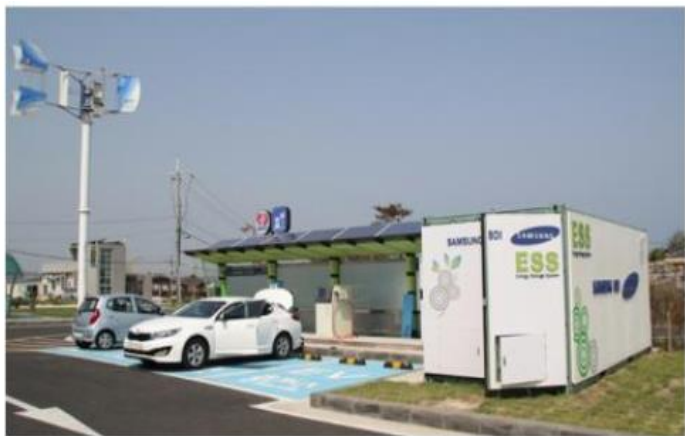
2009 SG 150kW ESS Demonstration
