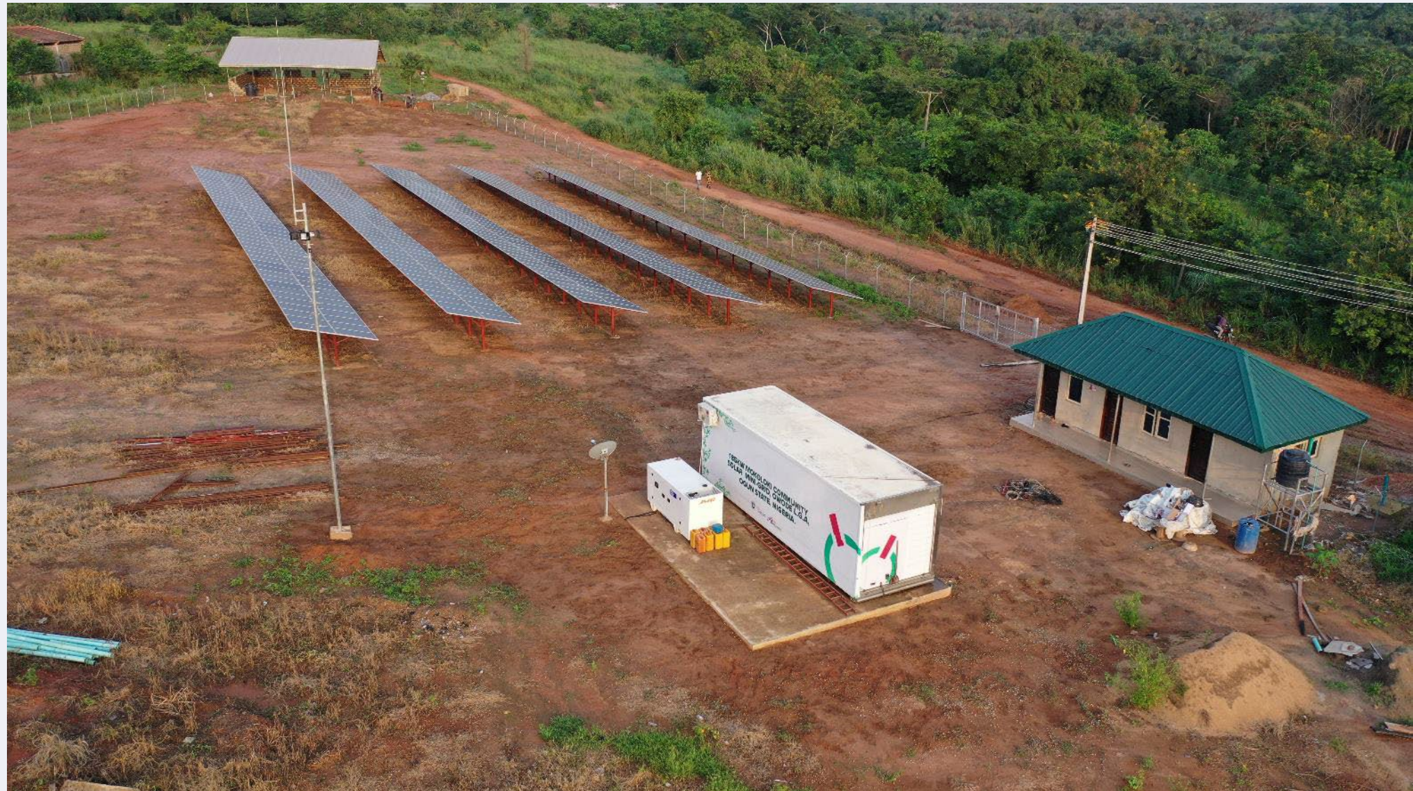
100 kWp solar PV, 192 kWh lead-acid battery, 88 kW diesel backup
