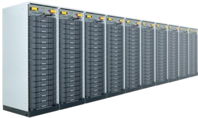
Battery Racks for ESS
