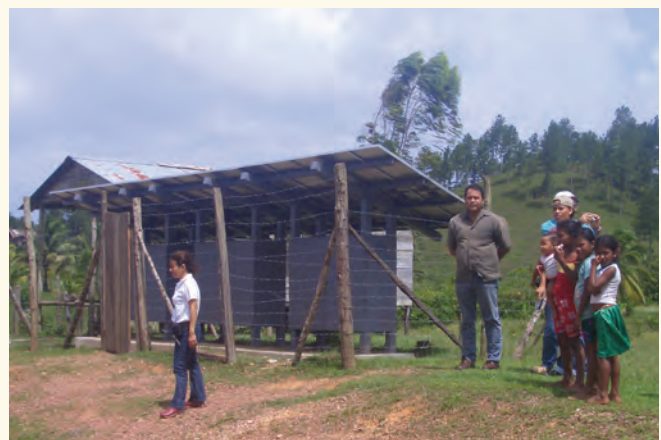
In Nicaragua's remote Atlantic Zone, 350 families benefit from 2-kW capacity, solar battery charging stations installed by the Offgrid Rural Electrification Project (PERZA).
