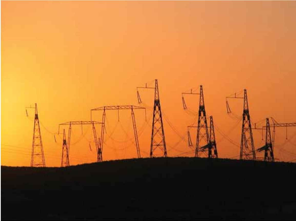
Power lines, Tajikistan.
